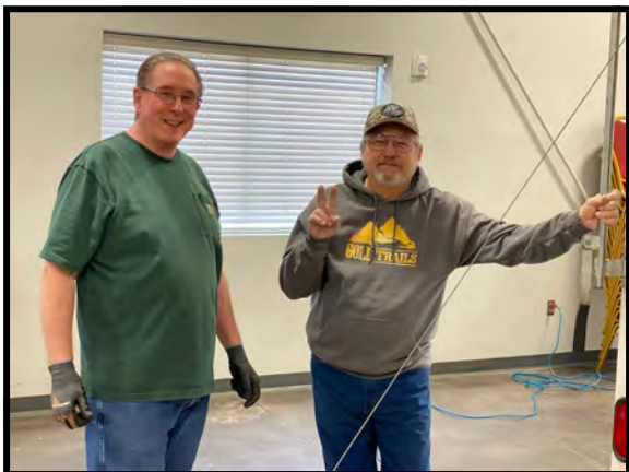
Clyde Ogg and Terry Anderson preparing to install the new UV lights in the fluorescent display. Terry's electrical experience made the installation a piece o' rock (I mean, cake).
